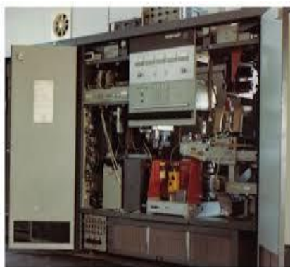
The AR5 Transmitter A photograph of the AR5 Transmitter, a large, open metal cabinet filled with various electronic components, including circuit boards, capacitors, and wiring. The cabinet is dark-colored and has a large door on the left side that is open, revealing the internal components. The components are densely packed and appear to be from the mid-20th century.
